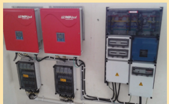
Monitors for Solar Plant
