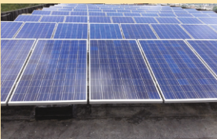
CMPDI roof top Solar Plant
